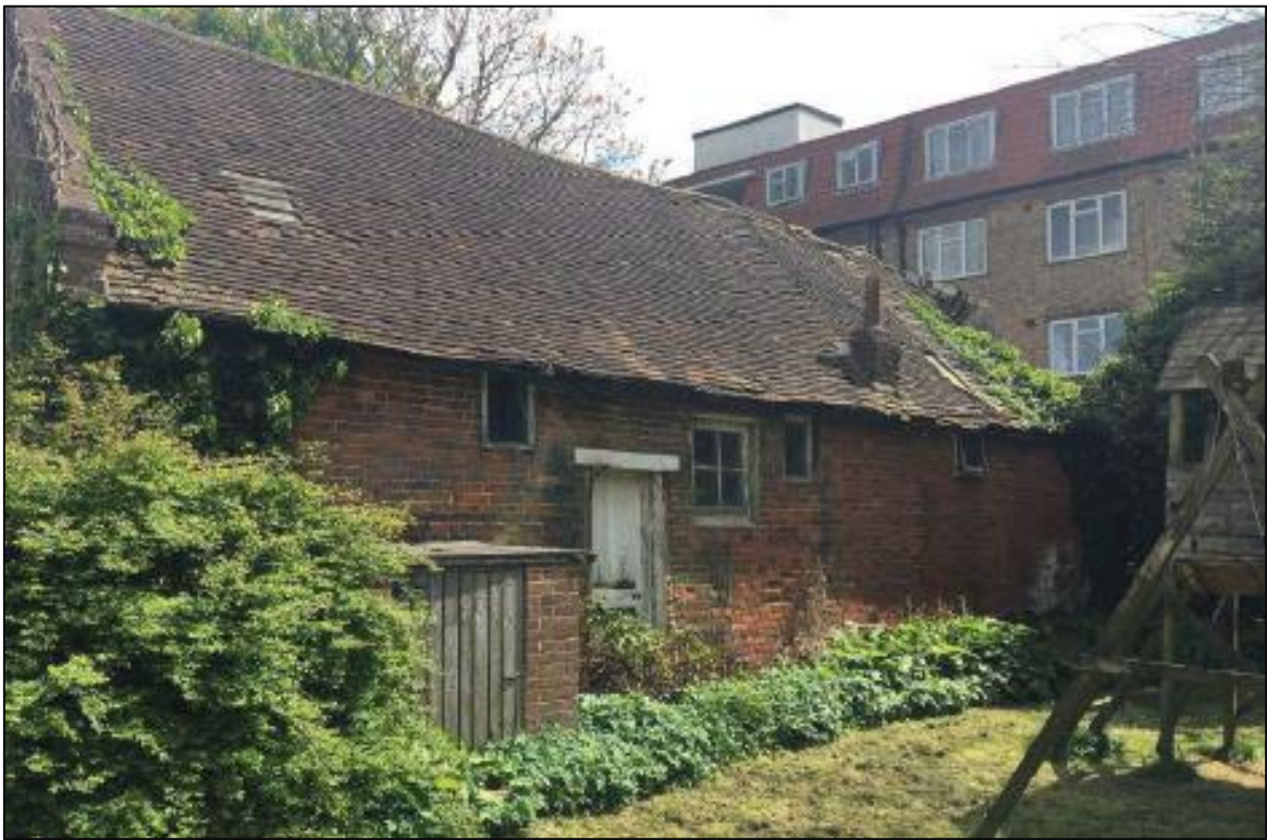
Fig2. Outbuilding prior to collapse
