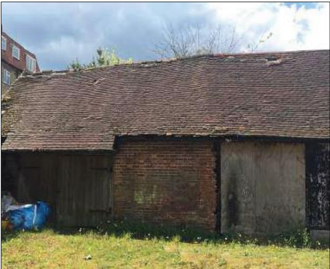
Fig3. Outbuilding prior to collapse
